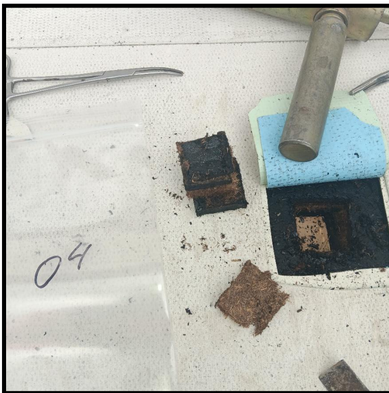
ASBESTOS Sample 04 old roof sample to clean wood ASBESTOS
