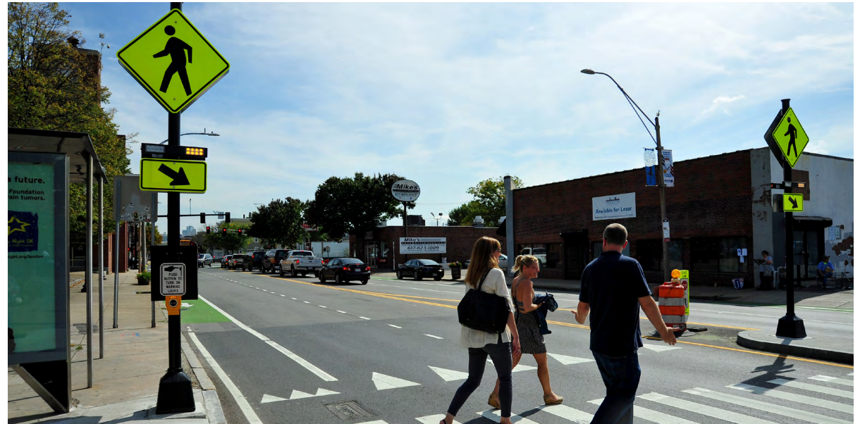
FIGURE 5-23 Rectangular Rapid Flashing Beacon (RRFB)
