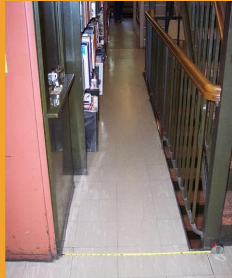
Patrons who use wheelchairs, walkers, strollers, or other adaptive equipment cannot access the stacks. In this photo, books are seen overflowing into the aisle, which is only 26” wide.
