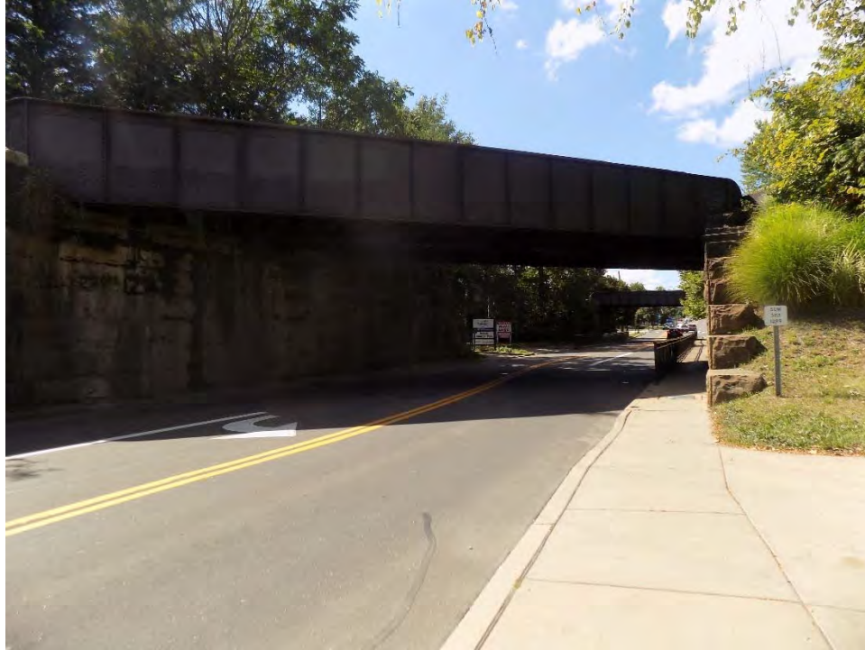
Figure 2: Sidewalk gap in constrained section of SR 303, looking west from Railroad access driveway
