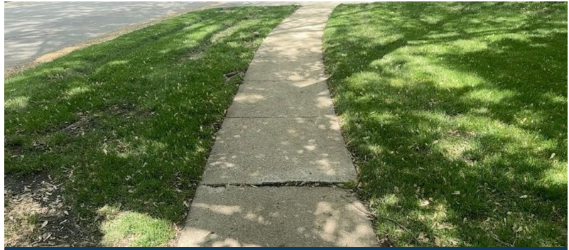
Example of sidewalk with tripping hazard where concrete is uneven.
